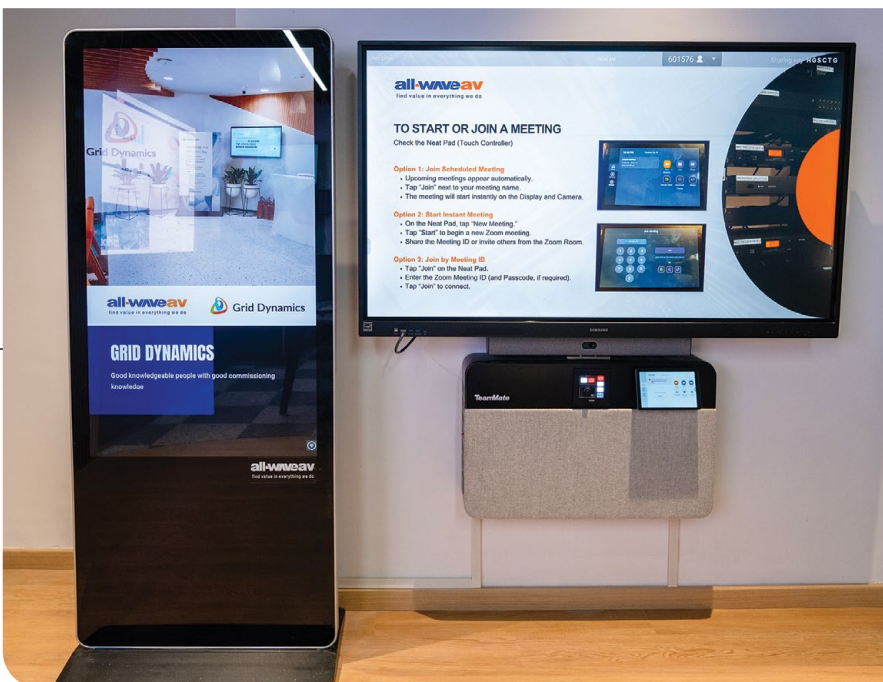
Huddle Space at the Workplace Technology Concept Centre is designed to bring together interactive displays, video conferencing, and active learning technology to serve small-group collaboration and training scenarios
