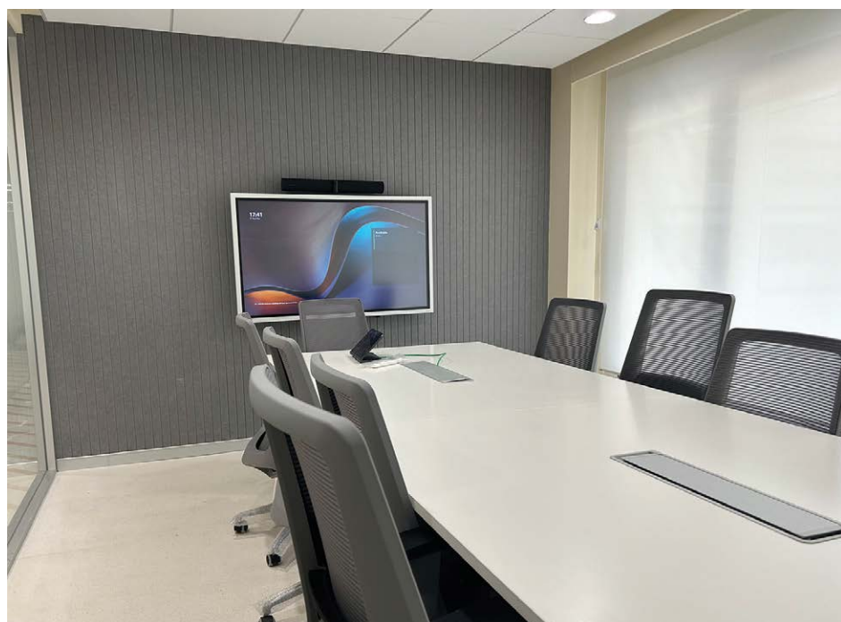
Conference room as installed by EYTE Technologies with bespoke AV Systems
