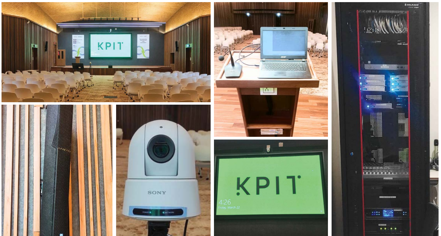
KPIT's Auditorium integrated with leading brands' comprehensive audiovisual solutions
